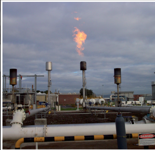
Mangere WWTP upgrade Fabricate and install, plant and piping Water Care Ltd, NZ
