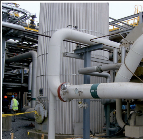
Southdown power station - Chiller and associated piping fabricate and install Mighty River Power Ltd, NZ
